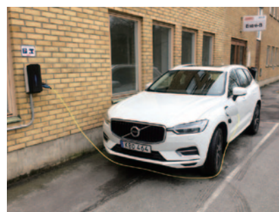
Power charging station
