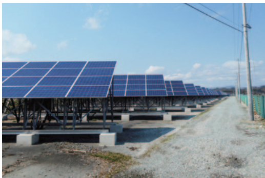
Murayama Solar Power Plant
