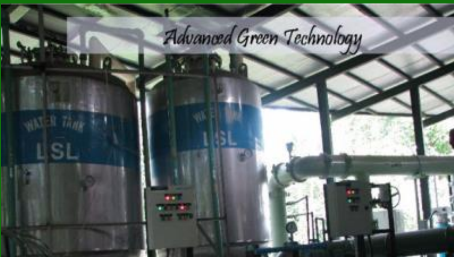
4 th Generation Heat Exchange Chiller System recovered heat waste is used for the hot water supply and hot water spa pool
