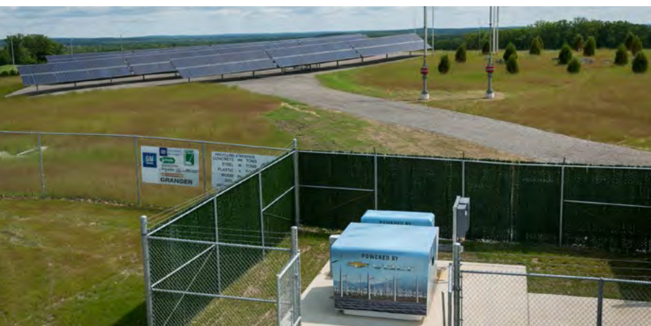
Used Chevrolet Volt batteries are helping keep the lights on at the new General Motors Enterprise Data Center at its Milford Proving Ground in Milford, Michigan. Five Volt batteries work with an adjacent solar array and two wind turbines to help supply power to the data center's administrative offices.
