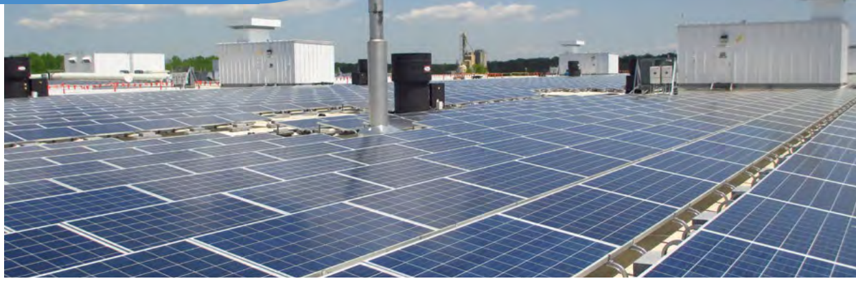
A 580 kilowatt solar array was recently added to the roof of our Baltimore Operation's e-Motor building, where electric motors and drive units for the Chevrolet Spark EV are built. This new array is made up of approximately 2,420 panels and covers 87 percent of the e-Motor building's roof.
