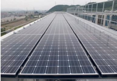
Solar panels at the Minase Research Institute
