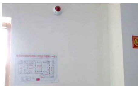
▲ Fire alarms and evacuation route maps
