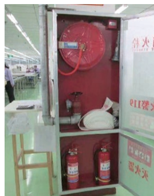
▲ Fire hydrants and fire extinguishers
