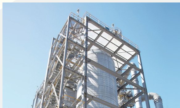
K/D HDS(Kero-Diesel Hydrodesulfurization Unit), which removes sulfur and nitrogen compounds, aromatic compounds, and metal components and increases specifications such as cetane number and fluidity.
