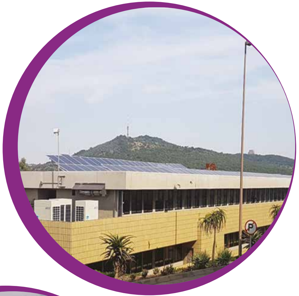
RR Maluleka Building rooftop solar farm
