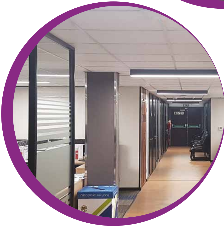
All-solar lighting inside RR Maluleka Building
