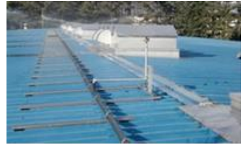
Running status of circulating roof spray system
