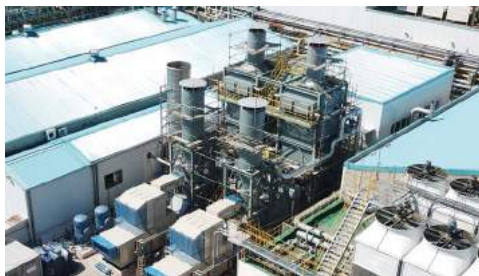
Co-generation Plant at the Ulsan Plant
