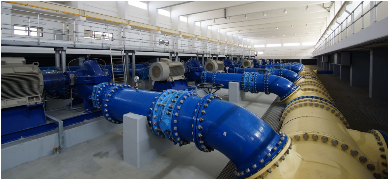
Sohar. Aspiracion Intermediate Pumping Station (Oman).
