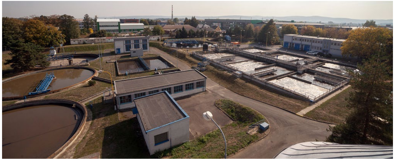
WWTP in Opava (Czech Republic).
