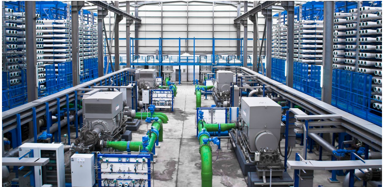
Desalination plant in Mostaganem (Algeria).
