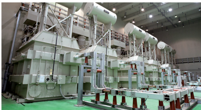
High voltage short-circuit transformer
