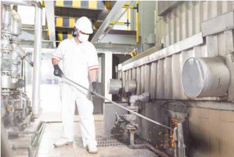
Steam generator that uses biomass from the soluble coffee extraction process, Coffee Business, Colombia.
