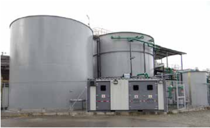
Wastewater treatment plant of the Cold Cuts Business.
