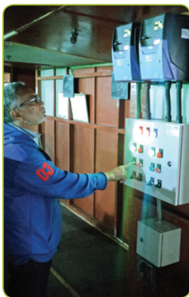
Newly installed Variable speed drivers operate by factory officer – Somerset Estate
