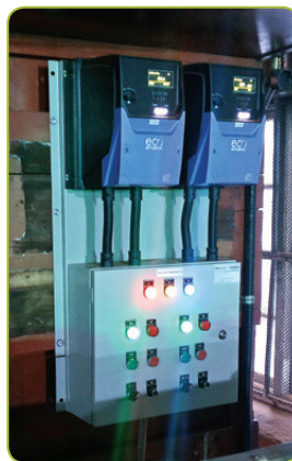
Newly installed Variable speed drivers for withering trough – Somerset Estate
