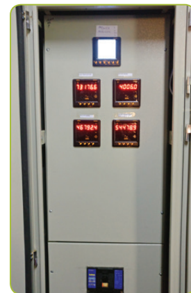
Newly installed Sub meters for monitor separate electricity consumption – Wategoda Estate
