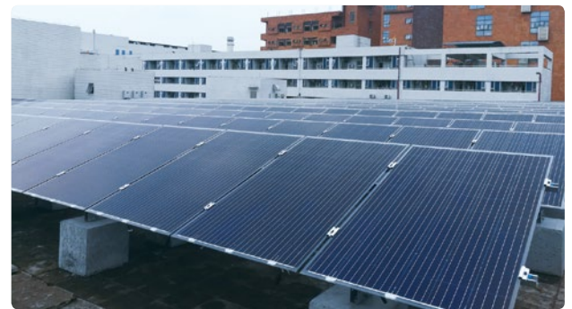
A solar power generating system(Tamron Optical(Foshan) in China)
