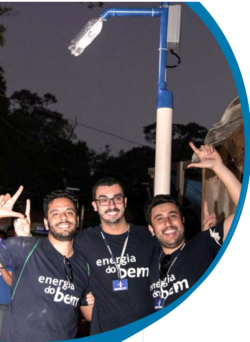
■ In an initiative that brought together social innovation and volunteer activity, the Energy Day of Good involved 74 volunteers in the installation of 30 lamp posts made from PET bottles and powered by solar energy, benefiting more than 2 thousand people in the community Vila Moraes (Sao Bernardo do Campo).
