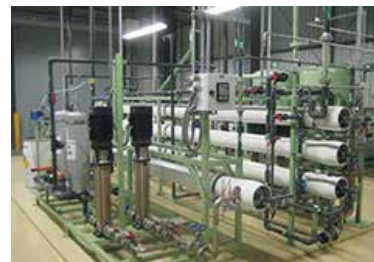
Filtration device using reverse osmosis membranes
