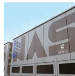
NAS battery which is the first megawatt-class electric energy storage system being utilized in the world
