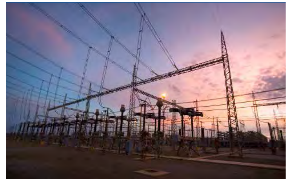
Our high-voltage transmission network links power stations and IPPs to our distribution network, which relays electricity to customers
