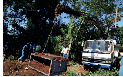
Recovery of a vandalised transformer in Kiambu County.
