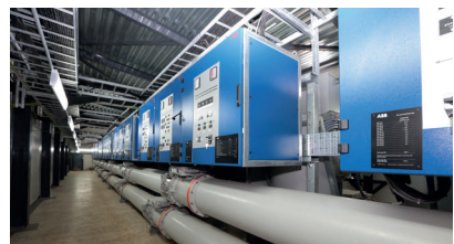
The new gas insulated substation at Juja Road, Nairobi.
