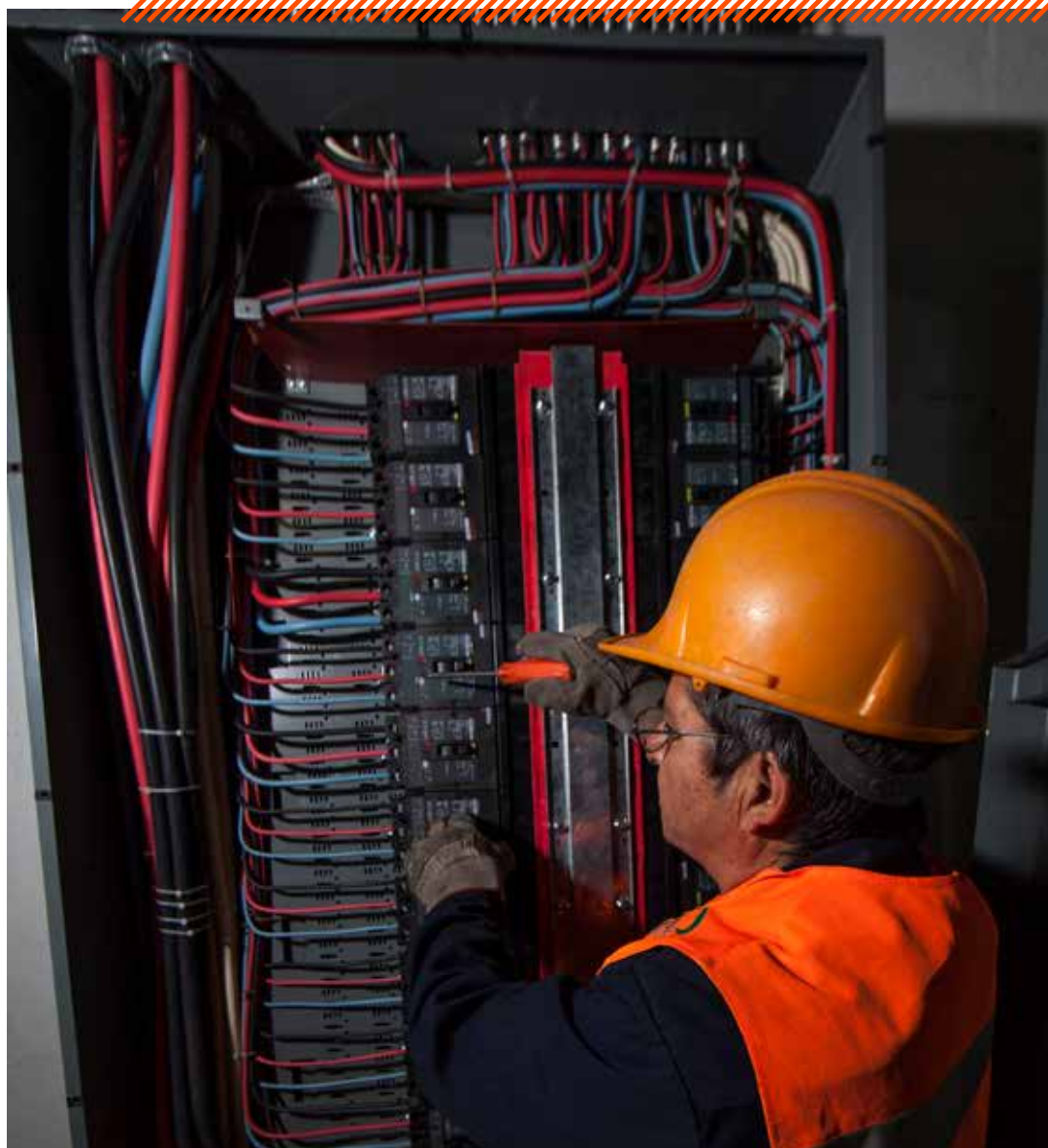
PHOTO: ELECTRIC MAINTAINANCE
