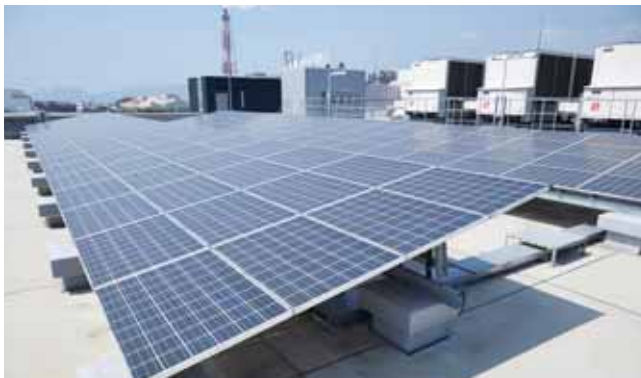
Solar Power Generation Facilities at Hikari plant
