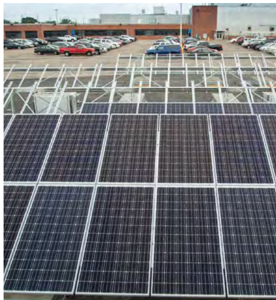
A new 800-kilowatt solar array at the Warren Transmission Operations is GM's largest solar installation in Michigan.
