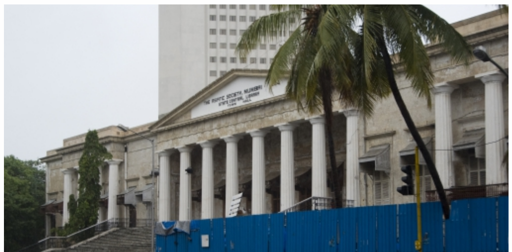
Restoration of the Durbar Hall at the historic Asiatic Society of Mumbai
