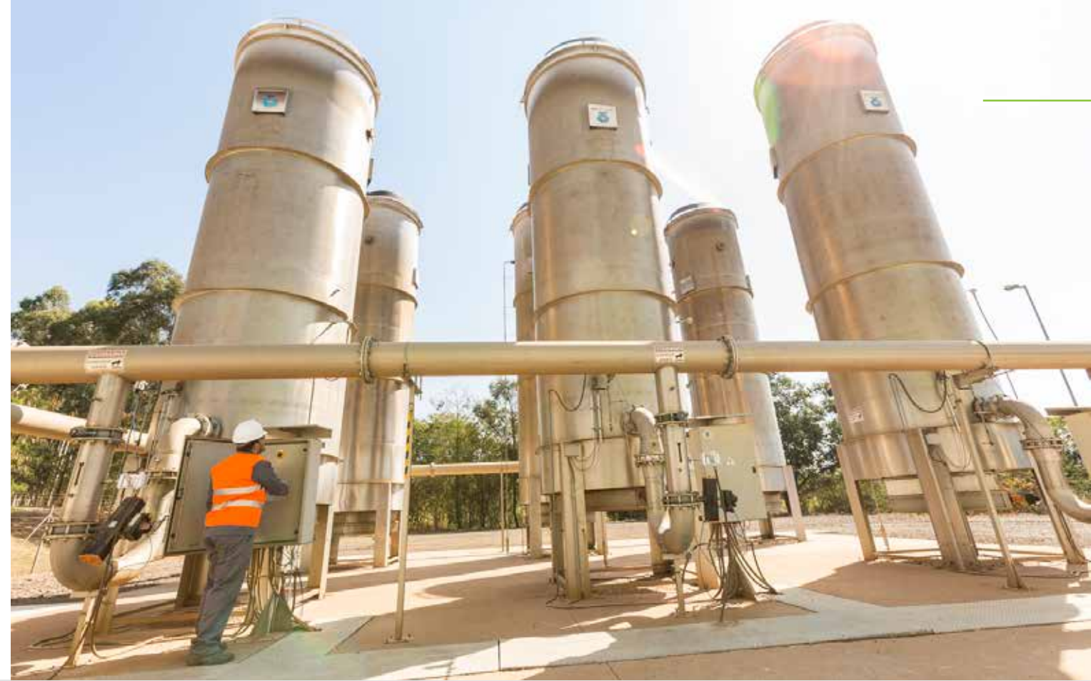
Biogas burning facility in Paulinia (SP)
