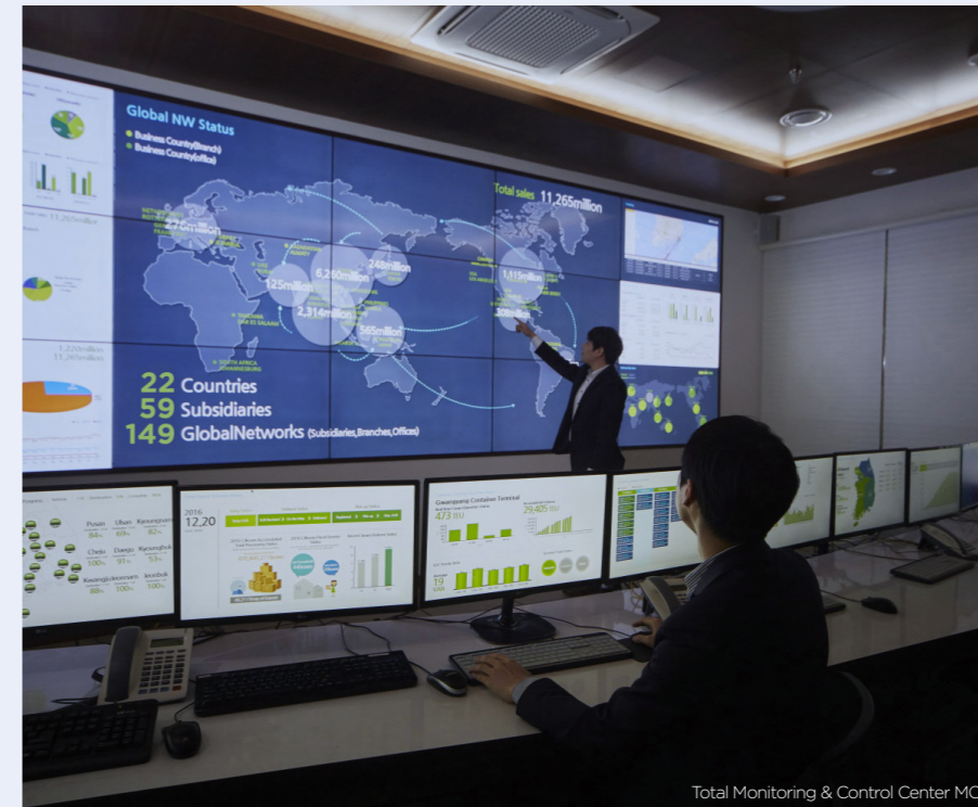
Total Monitoring & Control Center MCC
