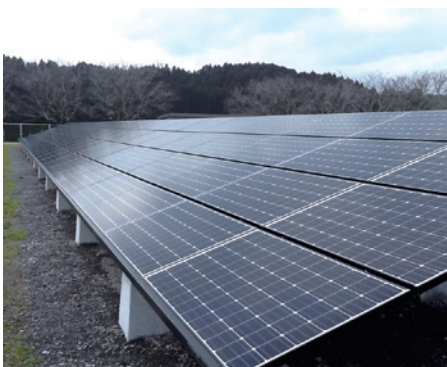
Solar panels installed on the grounds of the Saito Factory
