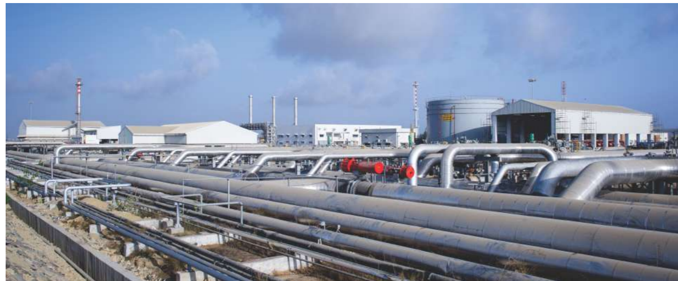
Bhogat Terminal, Gujarat – Cairn Oil and Gas business
