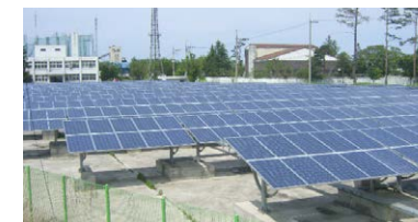
Gangneung PV Plant
