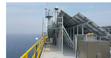
Maritime Safety Communication Facility
