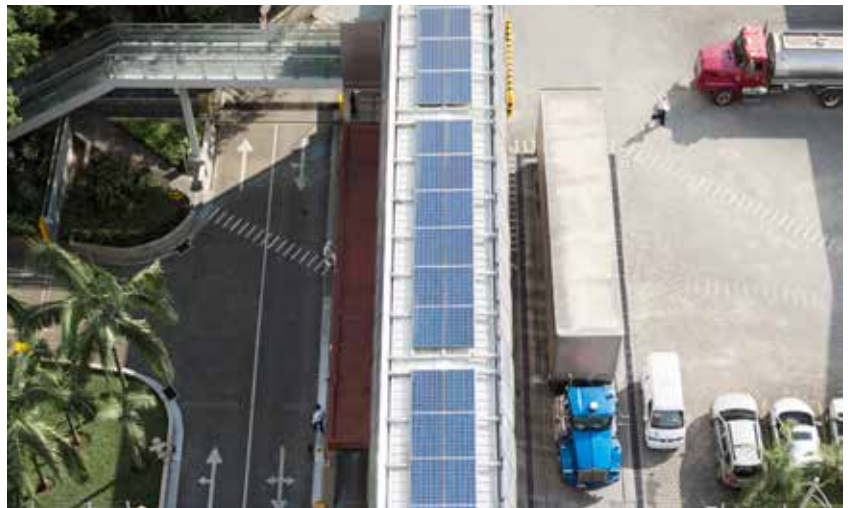
Photovoltaic solar panels, Colcafé Medellín.
