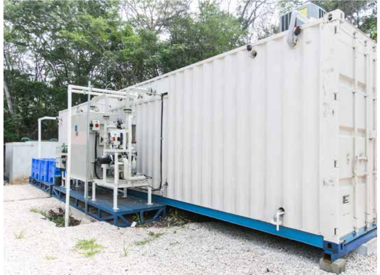
Desalination plant in Reserva Conchal
