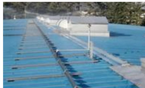
Running status of circulating roof spray system
