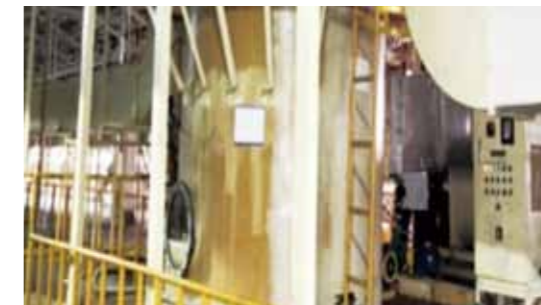
Improved the dust collectors installed at the pre-treatment equipment at paint shops of the Asan Plant
