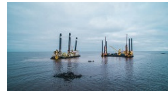
Dredging work at the sea area in front of Hanhikivi headland in fall 2016.
