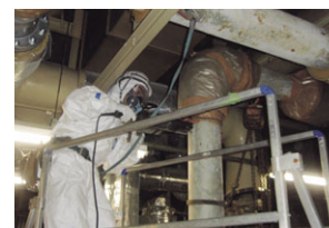
Confirmation of protective equipment and operational status
