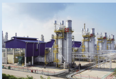
Petronas Penapisan (Melaka) Sdn Bhd Cogeneration Plant (Malaysia)
