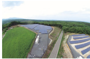
Large-scale photovoltaic power generation systems
