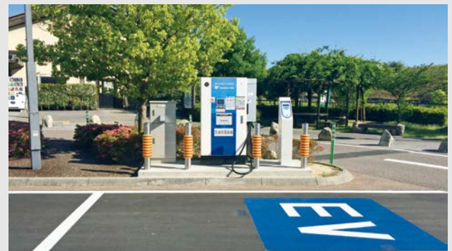
An example of an express charging station that Japan Charge Network has installed (Minokamo Service Area)
