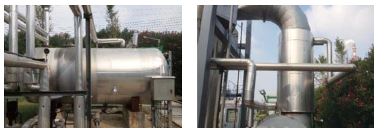
New hot water tank (left) and heat exchanger (right) to recycle waste heat
