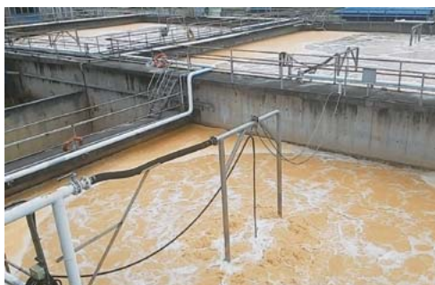
Wastewater treatment facility (DIC (Malaysia) Sdn. Bhd.)
