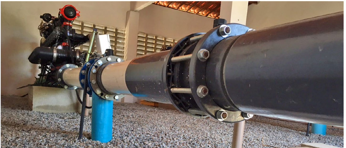
Our pumphouse with Netafim equipment for the distribution of water and fertilizers
