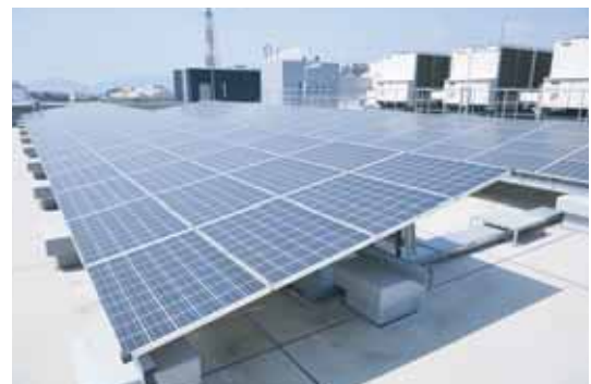
Solar power generation facilities at Hikari plant
