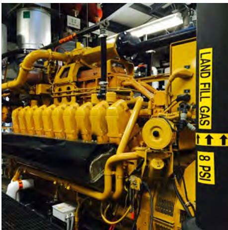
Landfill gas generators can provide up to 43 percent of electricity at our Fort Wayne Assembly Plant.
