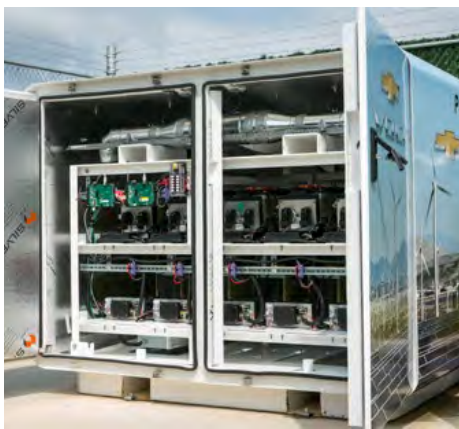
Five used Volt batteries help to power the GM Enterprise Data Center in Milford, Michigan.
