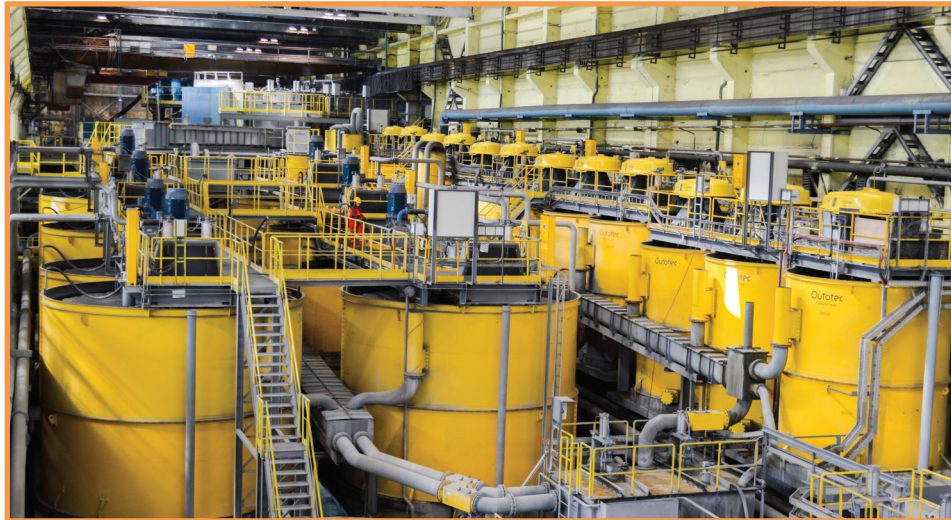
Flotation Department at the Asarel Flotation Plant
