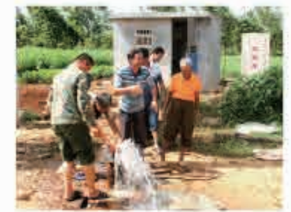
Wells for Acid Areas
