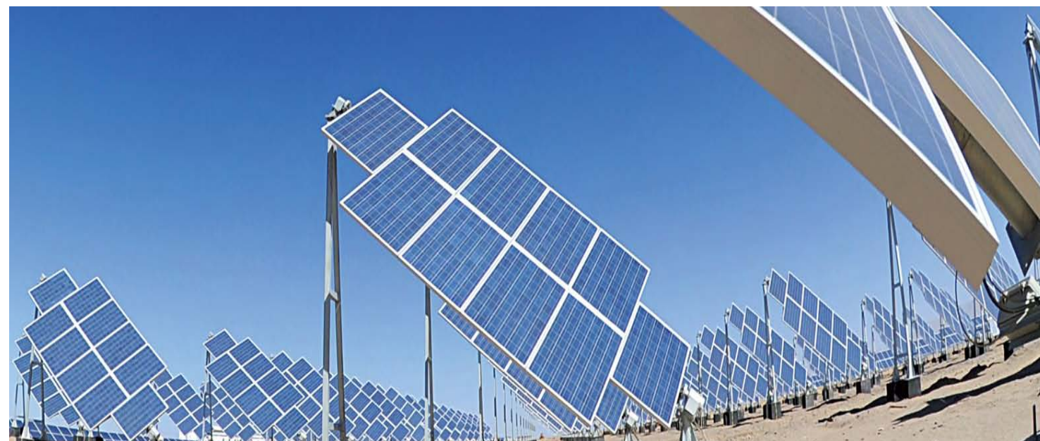
Golmud PV Project
