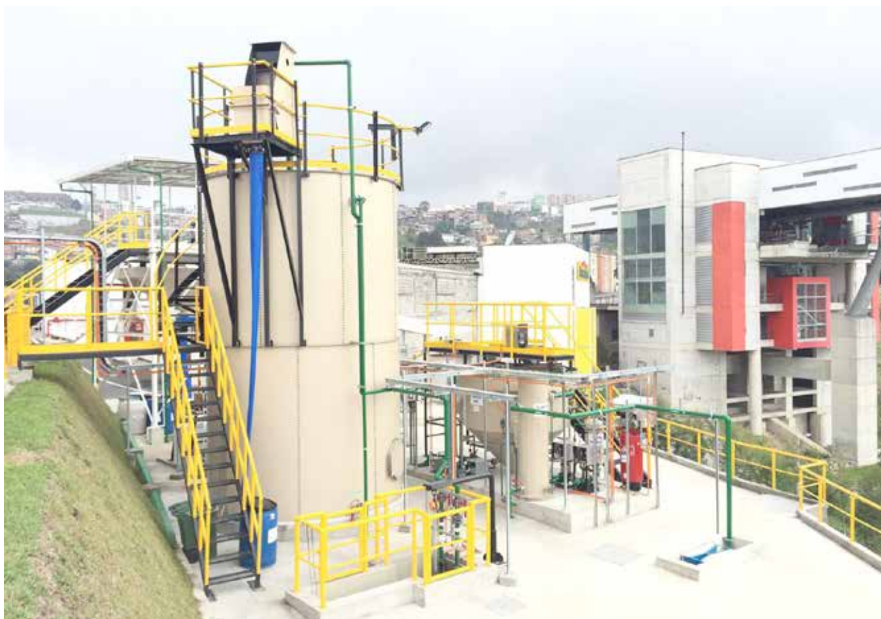
Waste water treatment plant of Ice Cream Business. Manizales, Colombia.
