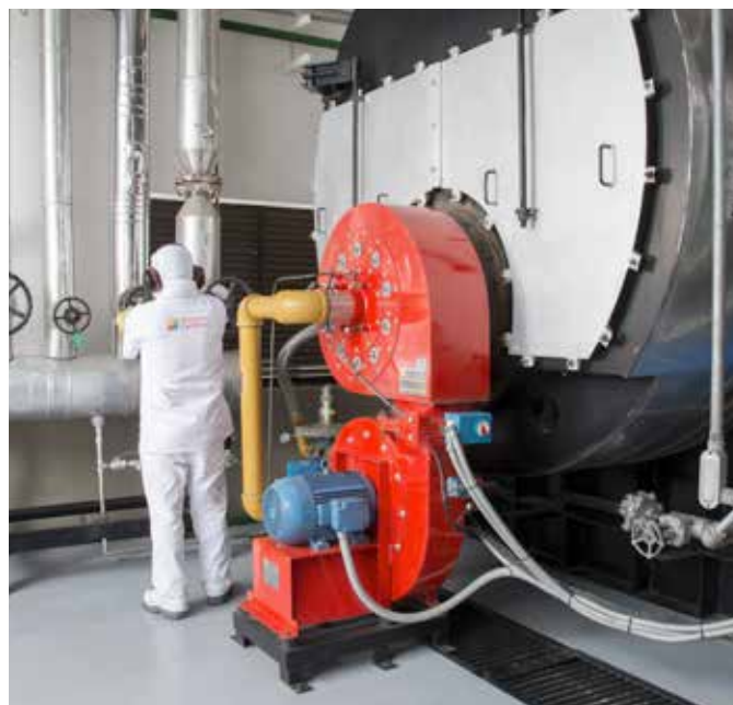
Boilers with cleaner energy. Meat Foods Plant in La Ceja, Colombia.
