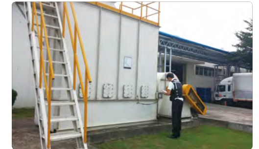
Inspection on air pollution prevention facilities
