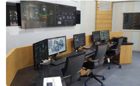
Automatic cooling and heating control system
