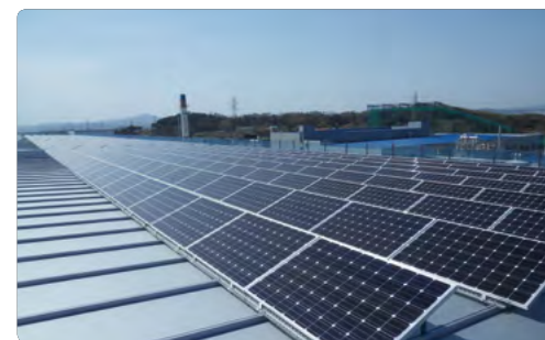
Photovoltaic power generation system
