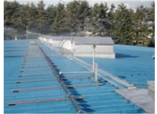
Running status of circulating roof spray system
