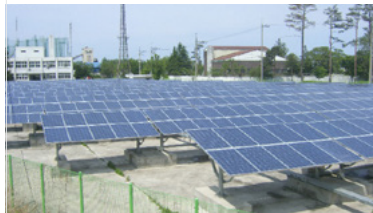
Gangneung PV Plant
