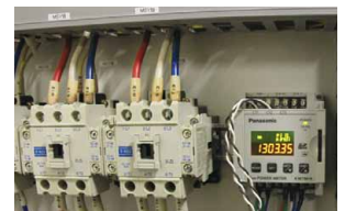
Streamlined electric power management sensor (Being used to measure the electric power consumption of the washing equipment at the Namioka Plant)
