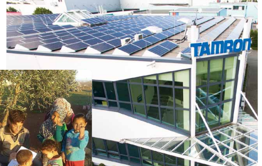
Rooftop PV panels at Tamron Europe GmbH
