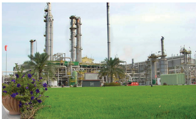
GPIC's Ammonia plant
