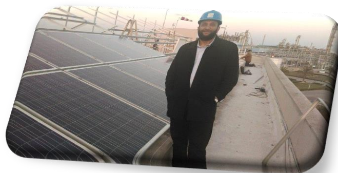
During the installation of SIDPEC solar station on the admin. Building in March 2015
