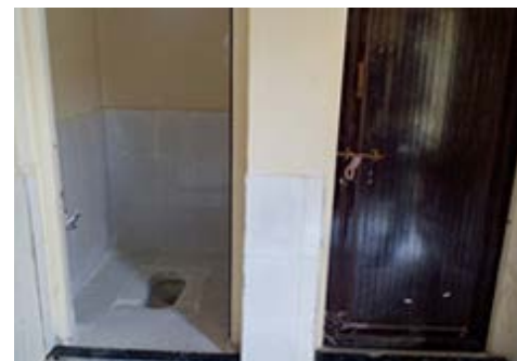
Toilet at Bolegaon Village
