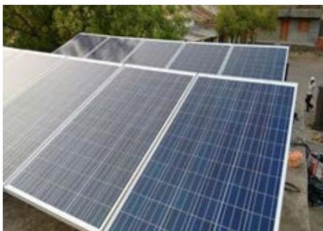
Solar Energy Panel at Bolegaon Village
