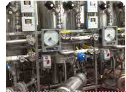
△ System that regulates chemical and water usage during cleaning processes at our facility in Carson, California.
